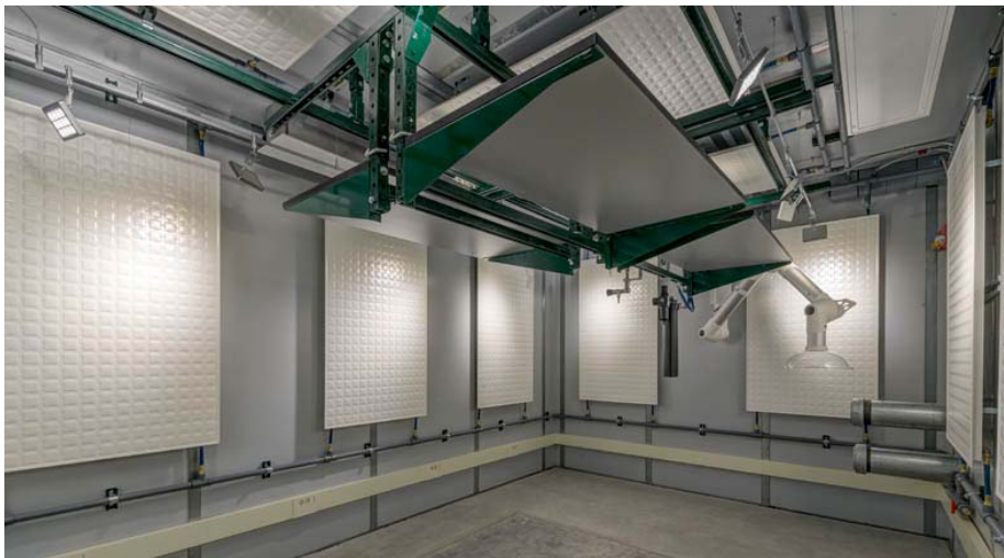
Ultra-low vibration chamber at ULVL with mass foundation, and RF shielding for the installation of a low vibration table.
