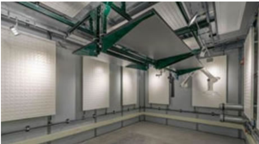
An ultra-low vibration chamber at ULVL with mass foundation, and RF shielding for the installation of a low vibration table.
